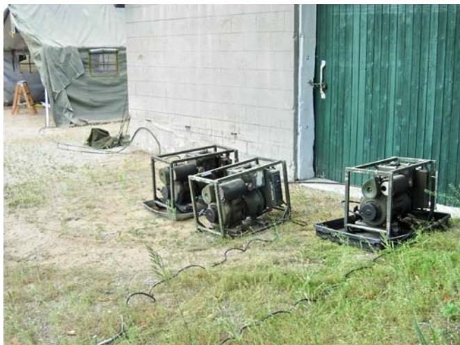
Generators to power the radio equipment
